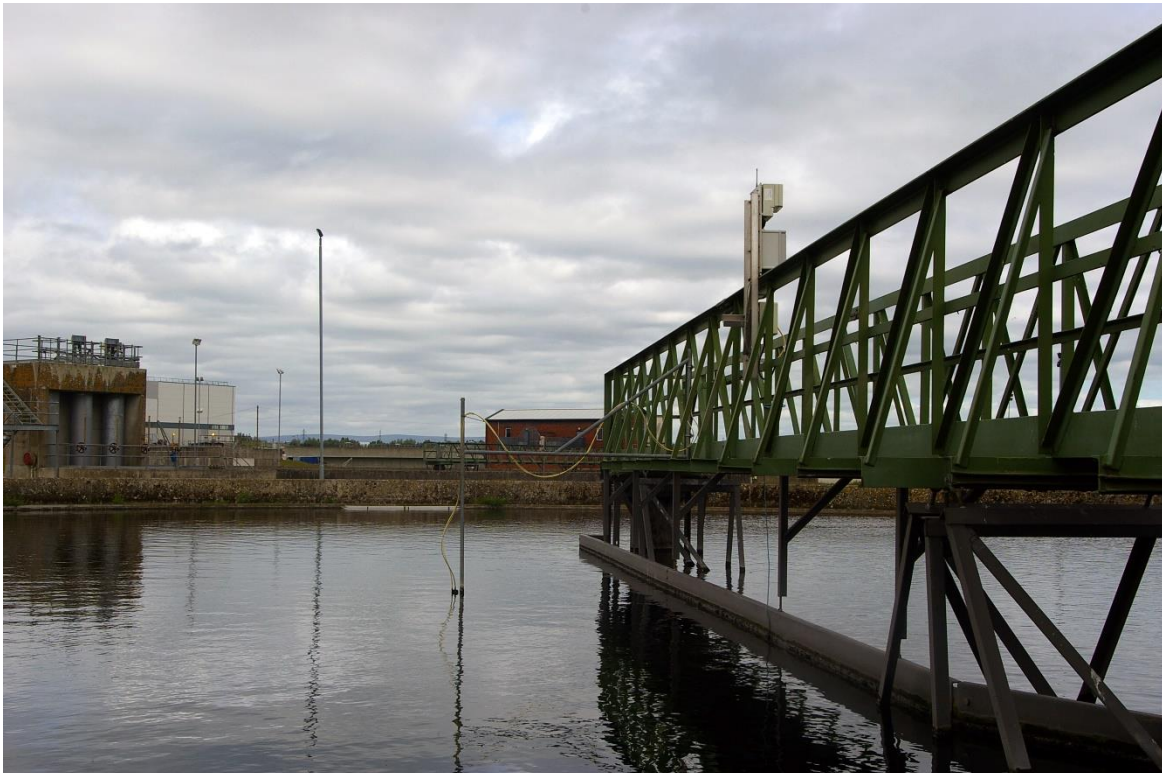
Figure 4 Avocet-9000 Outstation Installation
